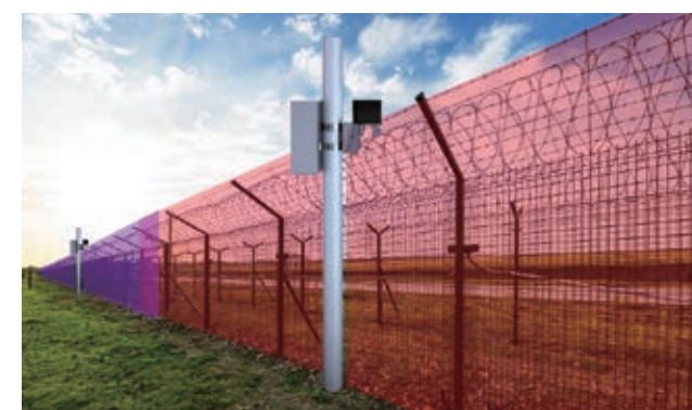
Airport Perimeter Security System
