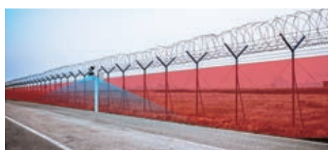
Airports Perimeter Security
